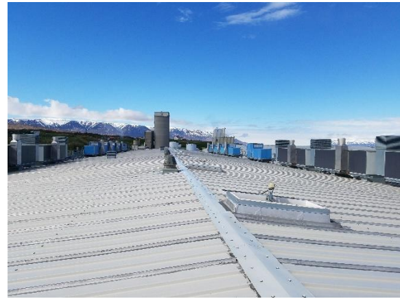
Picture 2-6: Exhaust units on the roof
